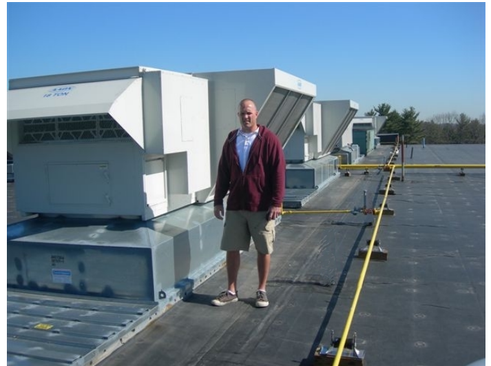
Custodian Tim Fournier comments there is no added maintenance for the energy recovery wheels.
